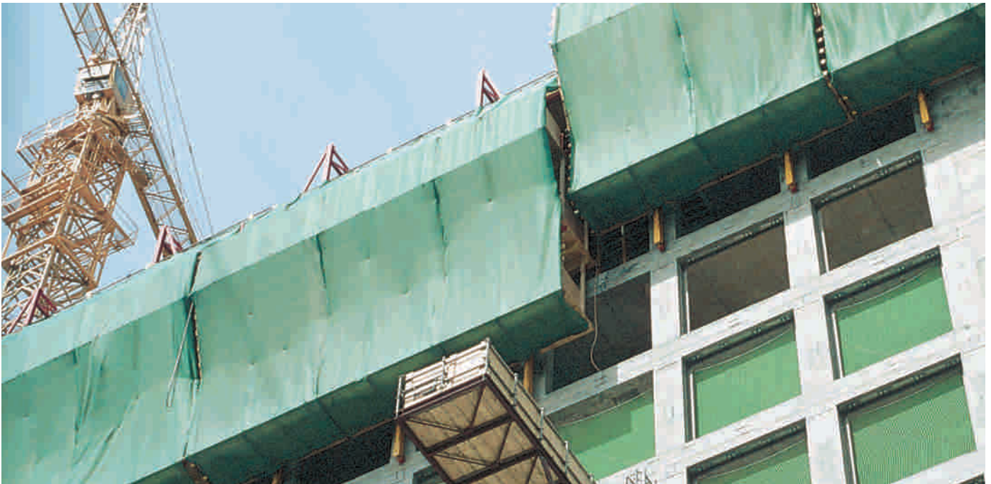
Side protection with close mesh heavy duty nets and air permeable PE panels during the building of the Japan Centre in Frankfurt. 1
