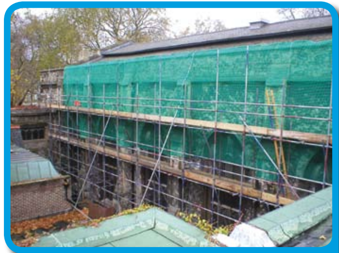
Debris Control Netting
