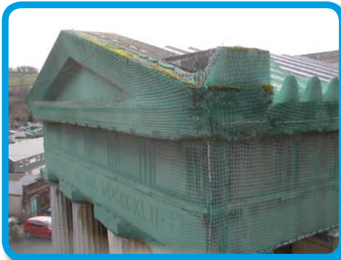
Debris Control Netting
