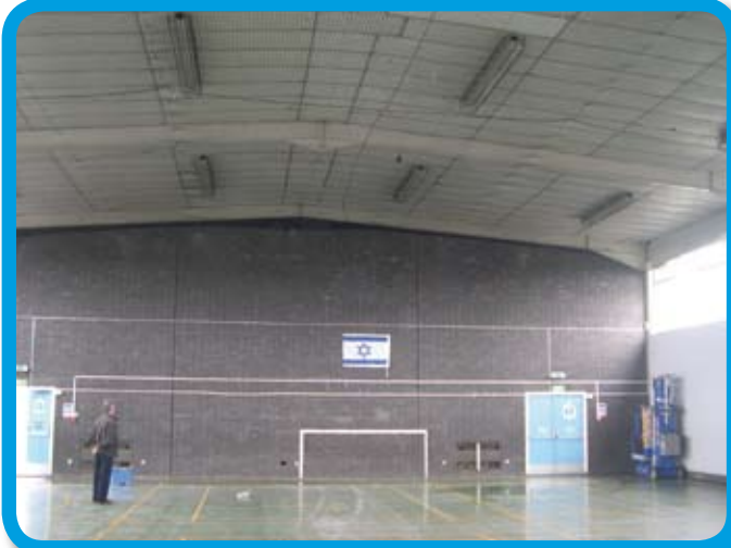
Roof Protection Netting
