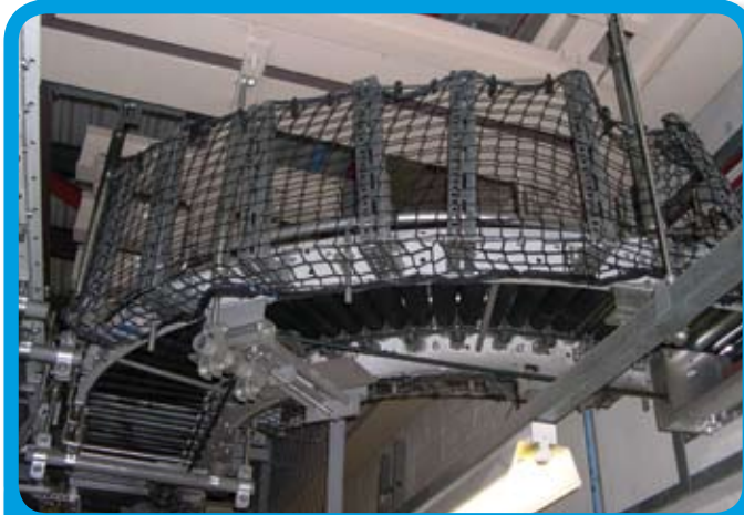
Conveyor - Catch Netting
