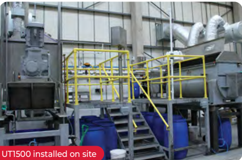
UT1500 installed on site
