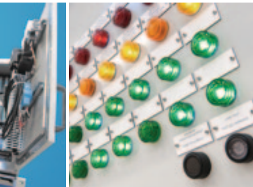
Control panel with STAHL series 8010/8082 signal lights and pushbuttons
