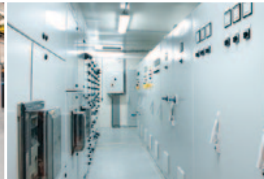
Containerized Low Voltage MCC, control panel and electrical heater thyristor panels
