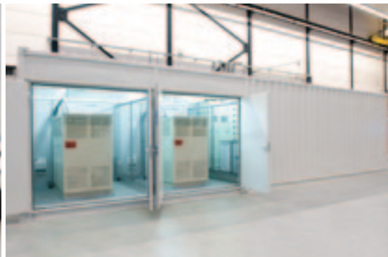
Containerized control building for Root Compressor including power transformers
