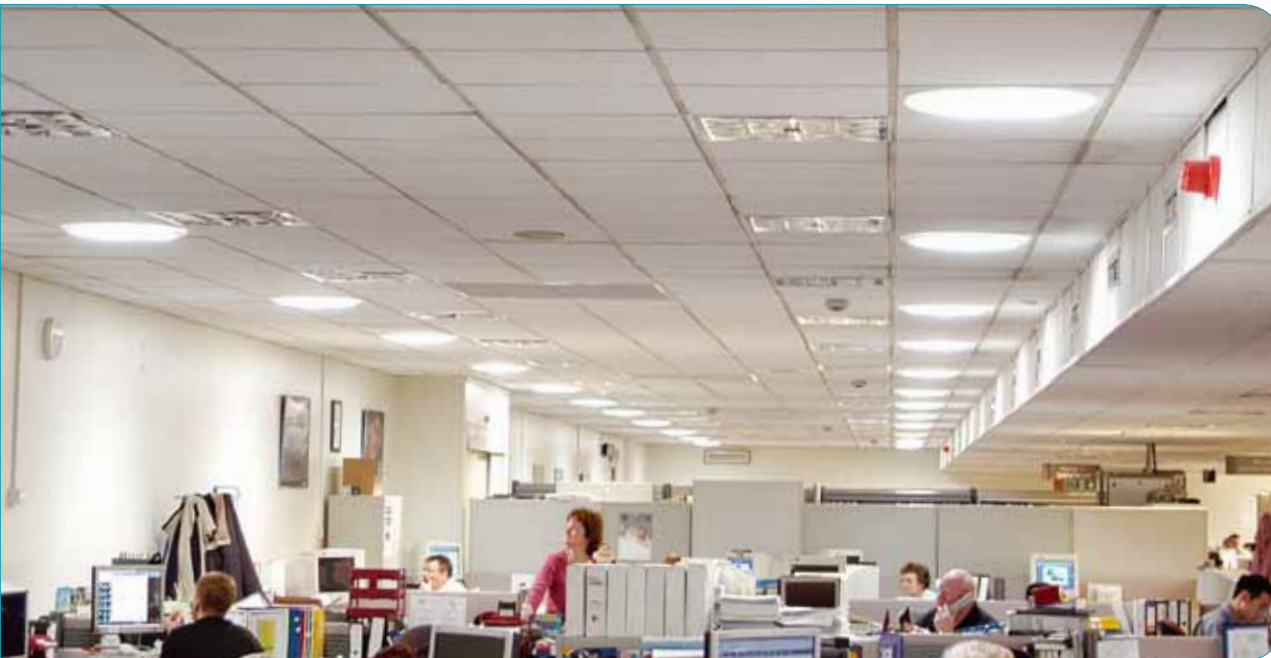
Above: Internal view of WINDCATCHER and SUNPIPE systems installed at the Daimler Chrysler offices in Milton Keynes
