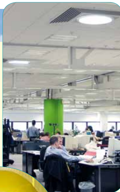
SUNCATCHER installations at the BMW head offices
