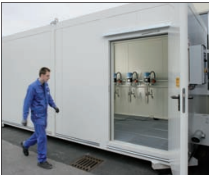
Figure on the left: Fire protection storage with T90 (90 Minute) door including door retaining device.
