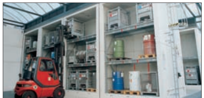
Large storage facility for new and used goods with a capacity of 2 x 72 tonnes of flammable or toxic liquids.
