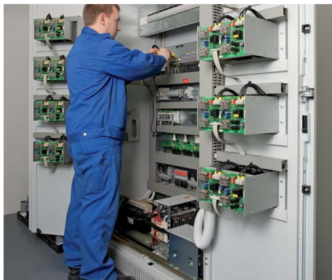
Final assembly of emergency power supply at the factory in Bad Oeynhausen
