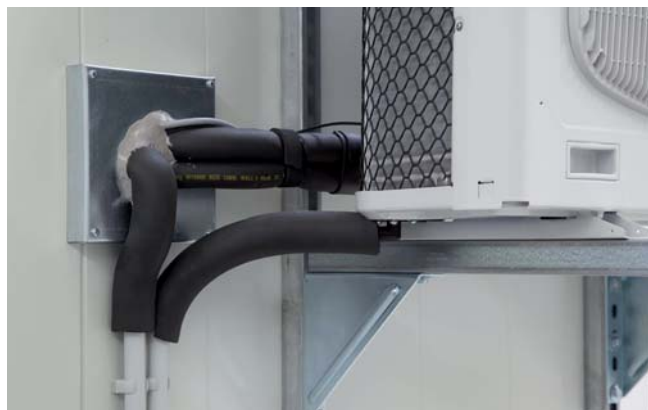
Fire-protected feedthrough glands of pipes in a side wall
