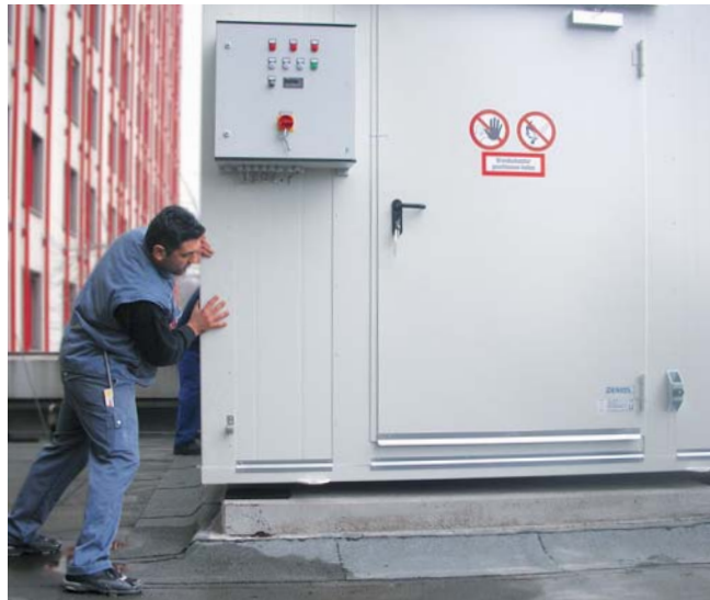
The technical room can be setup right on the roof of the hospital
