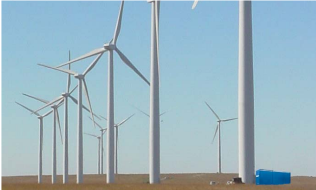
Container with switching station on wind turbine
