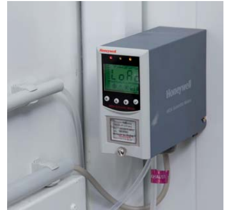
Gas warning detector
