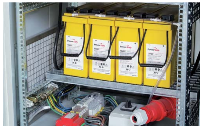
Battery-backed emergency power supply
