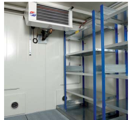
Ventilation system and shelves with sumps
