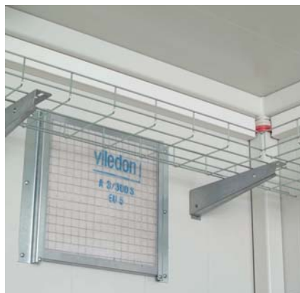
Cable tray and inlet opening with coarse filter
