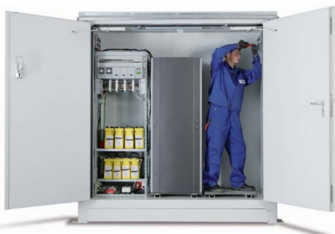
Room with radio and emergency power technology/equipment
