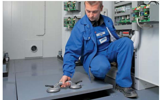
Double floor for laying cable
