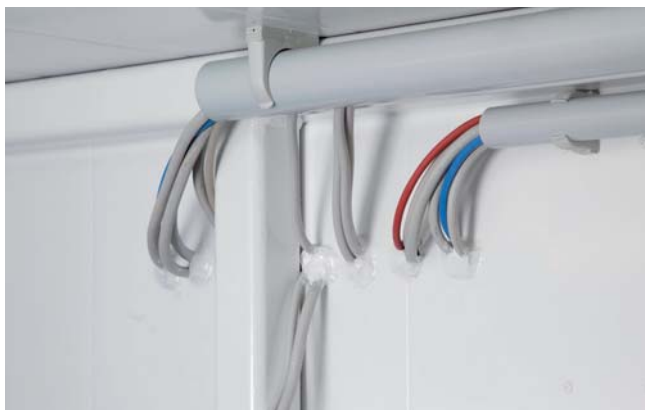
Fire-protected feedthrough glands of cables in a side wall
