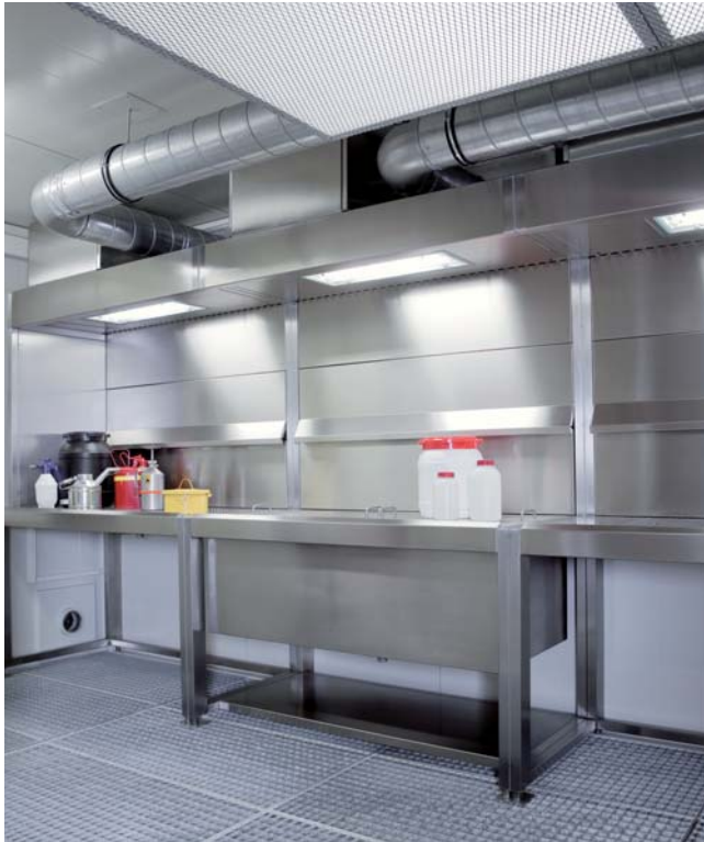
Interior design with vented workbenches for optimum personal protection
