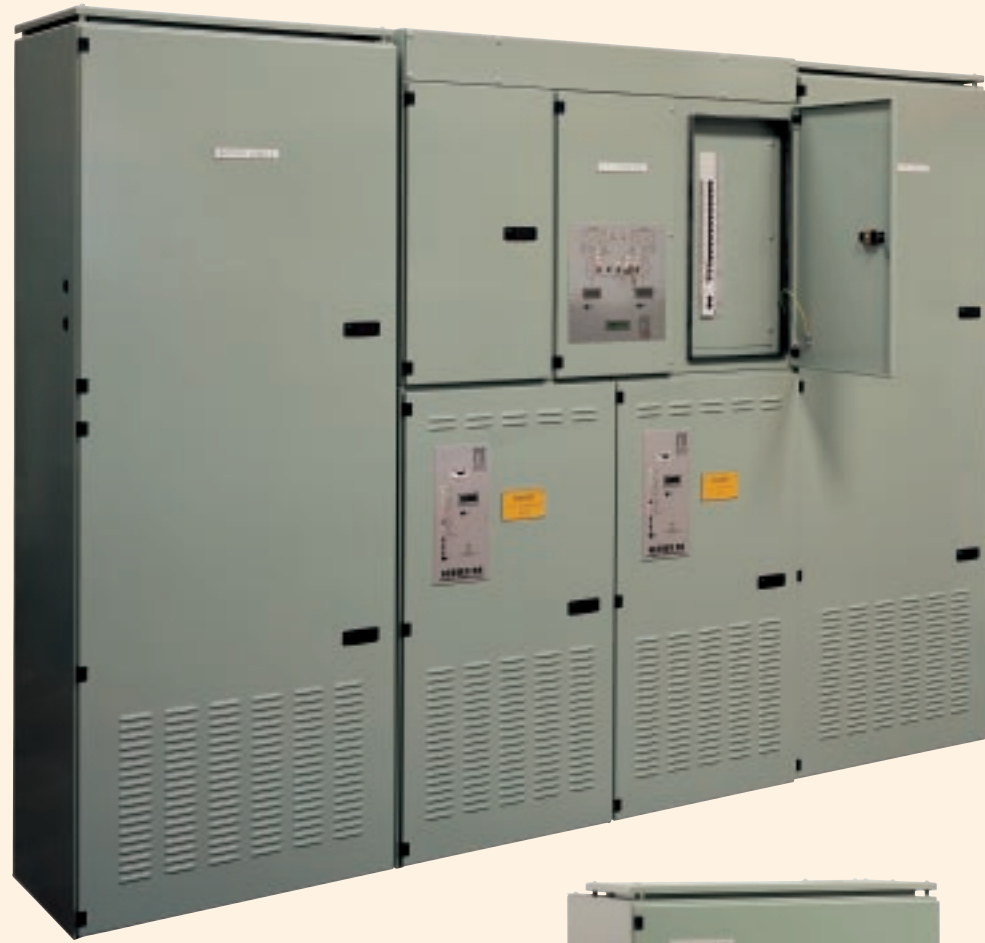
Dual 110V charging system with segregated distribution for the rail industry
