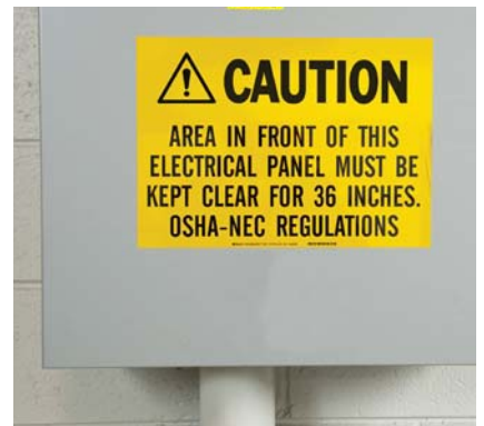
Hazard warning signs
