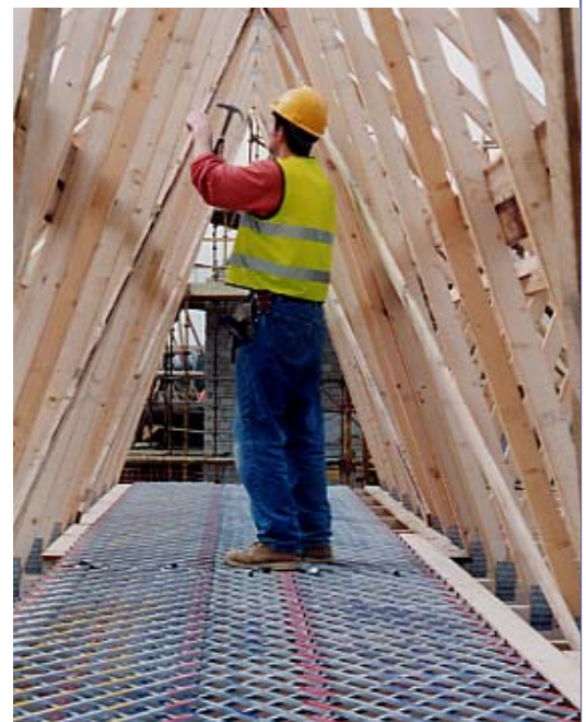
Providing a quick and easy safe working "platform" or deck across the ceiling rafters of trusses
