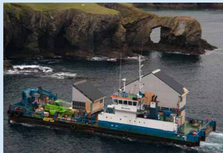
Top: Work continues assembling the pre-constructed pods Centre: The site as seen looking towards the sea Bottom: Pods arriving by sea aboard the MCS Ailsa
