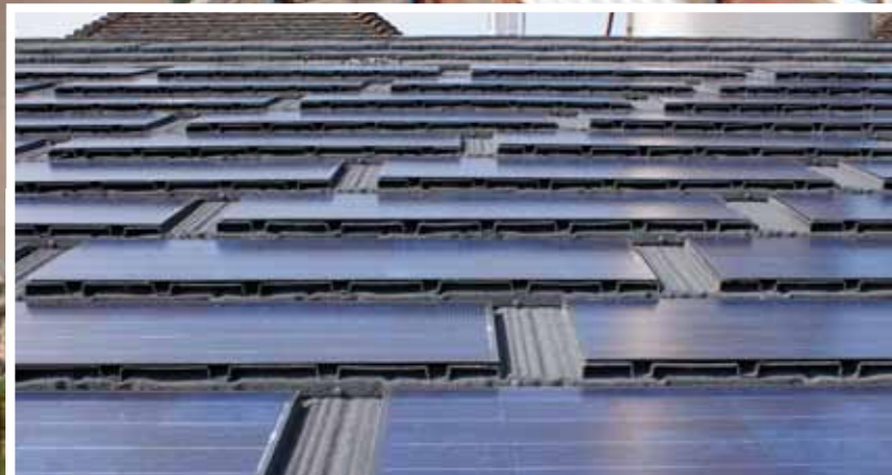
200 Photovoltaic panels on the south-facing roof supplies energy back to the National Grid
