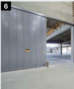
6 Fire sliding doors
