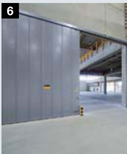
6 Fire sliding doors
