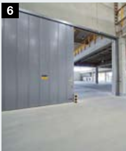
6 Fire sliding doors
