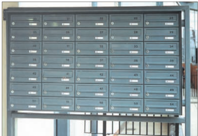
Internal mounted bank with engraved numerals and rectangular frame 20-311 with crossbeam.
