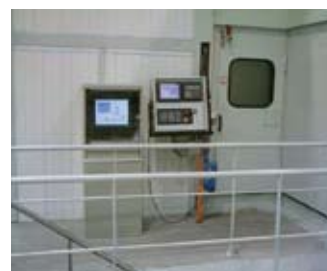
Supervision PC and CNC board
