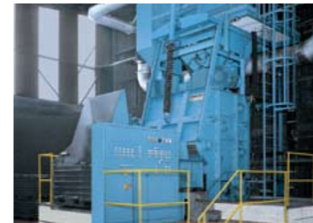
ST-28 in a foundry
