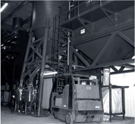
Media silo with pressure vessel
