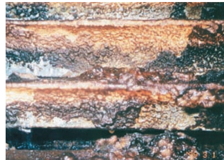
Heavy cooking grease contamination
