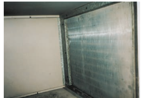
Heating coil returned to efficient operation
