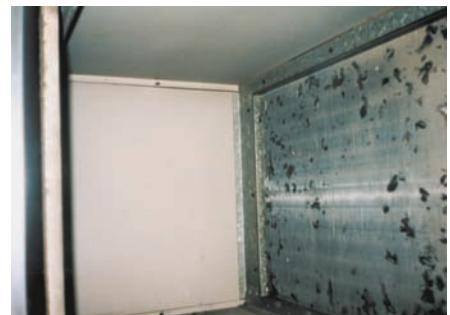
Contaminated heating coil
