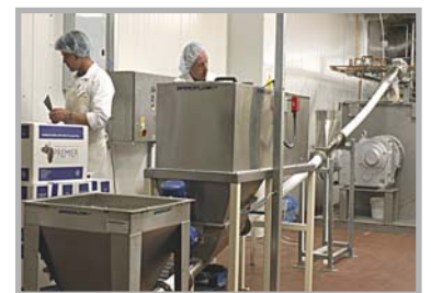
Multiple inlets and/or outlets.
