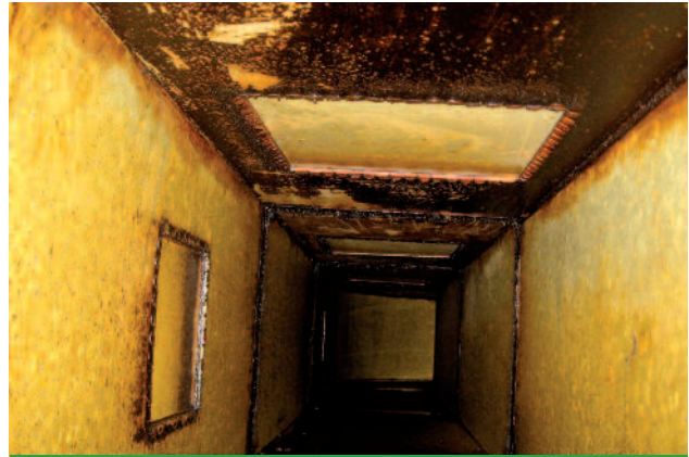
Kitchen extract duct before cleaning
