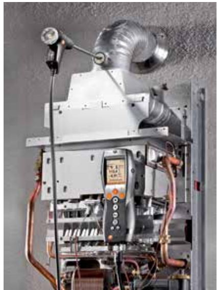
Fig. 8: A flue gas analyzer, e.g. testo 330, is essential for carrying out adjustments
