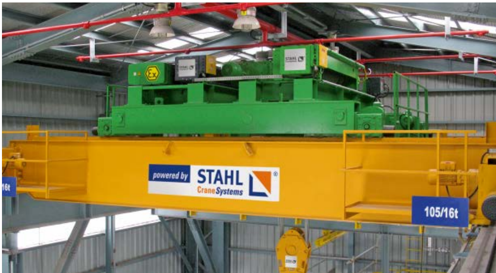
Explosion-protected wire rope hoists in twin design with auxiliary hoist facilitate compressor maintenance in a hydrogen liquefaction plant.
