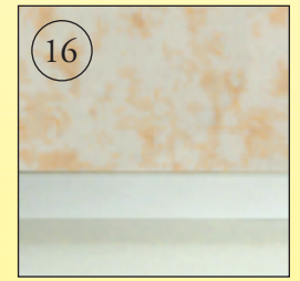
16 Bed cladding in Sealux-N on strip
