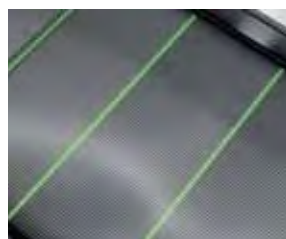
Under step demarcation lighting
