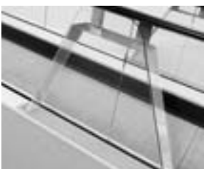
Anti-climb barrier (EN115-1:2008 + A1:2010 requirement)
