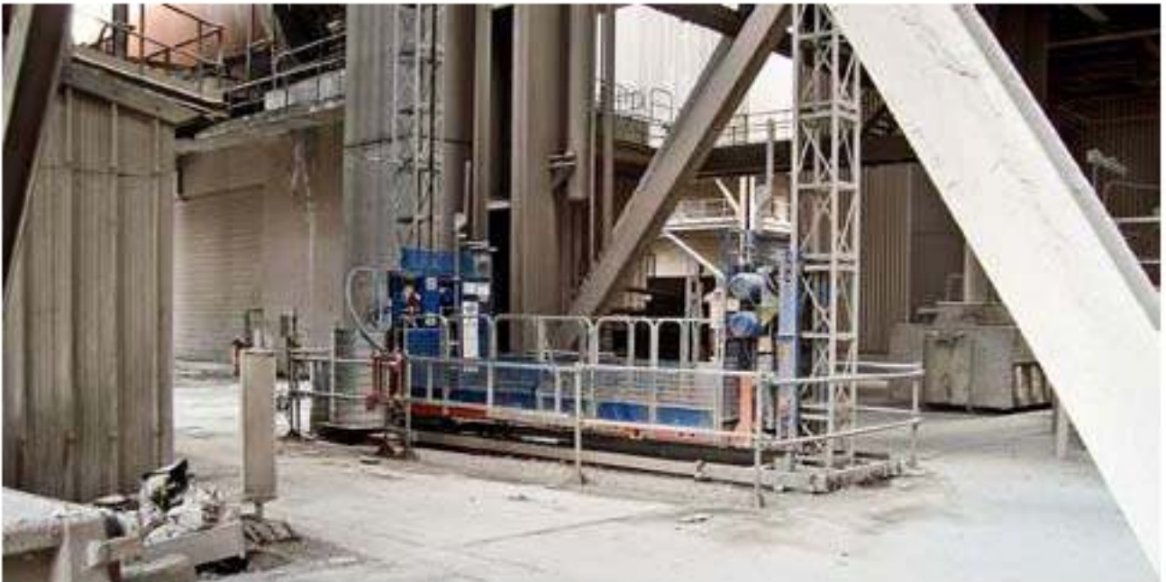
Another example of a project: CCB, Belgium Twin mast HEK TPM 4000T used for maintenance work on a cement factory. Client: CCB. Location: Doornik, Belgium.
