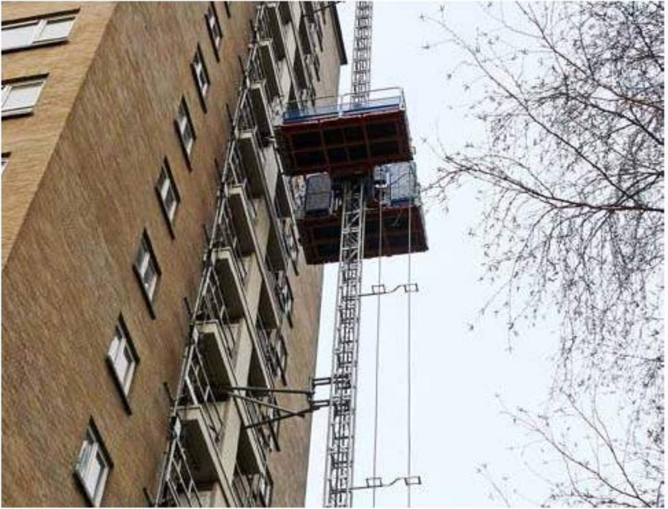
Example of a project: Brebuild, Belgium Two HEK TPM 1300SD on one mast used for a renovation project. Contractor: Brebuild. Location: Antwerp, Belgium.
