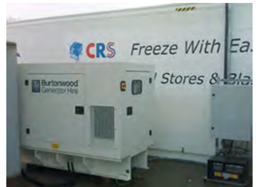
Generators on hire for the NHS
