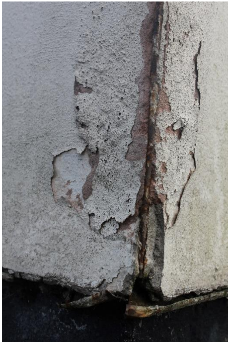
Images 3 - 5: The use of steel beading can degrade building aesthetics over time, due to visible rusting and potential damage to the render.
